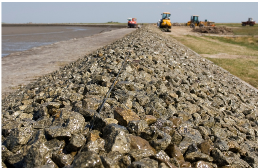
Figure 1. Polyurethane bonded aggregate (PBA) revetment (photo: BASF)
