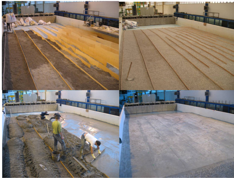
Figure 4. Bathymetry construction: First gravel padding along the longitudinal profiles, concrete flushing and bathymetry completed.
