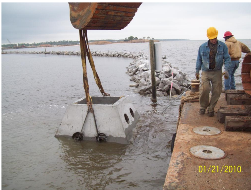
Figure 8 . Placement of the first “Wave Attenuation Device” or WAD, which was part of the porous breakwater system. In the background is the eastern end of the breakwater which was all rock.
