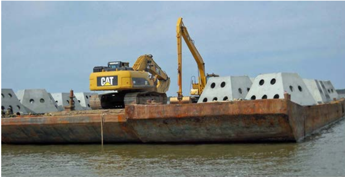
Figure 9. The “Wave Attenuation Devices,” or WADs, used in the Little Bay project breakwater. The WADs used here were truncated, four-sided, pyramid-shaped concrete units with circular holes in the faces.
