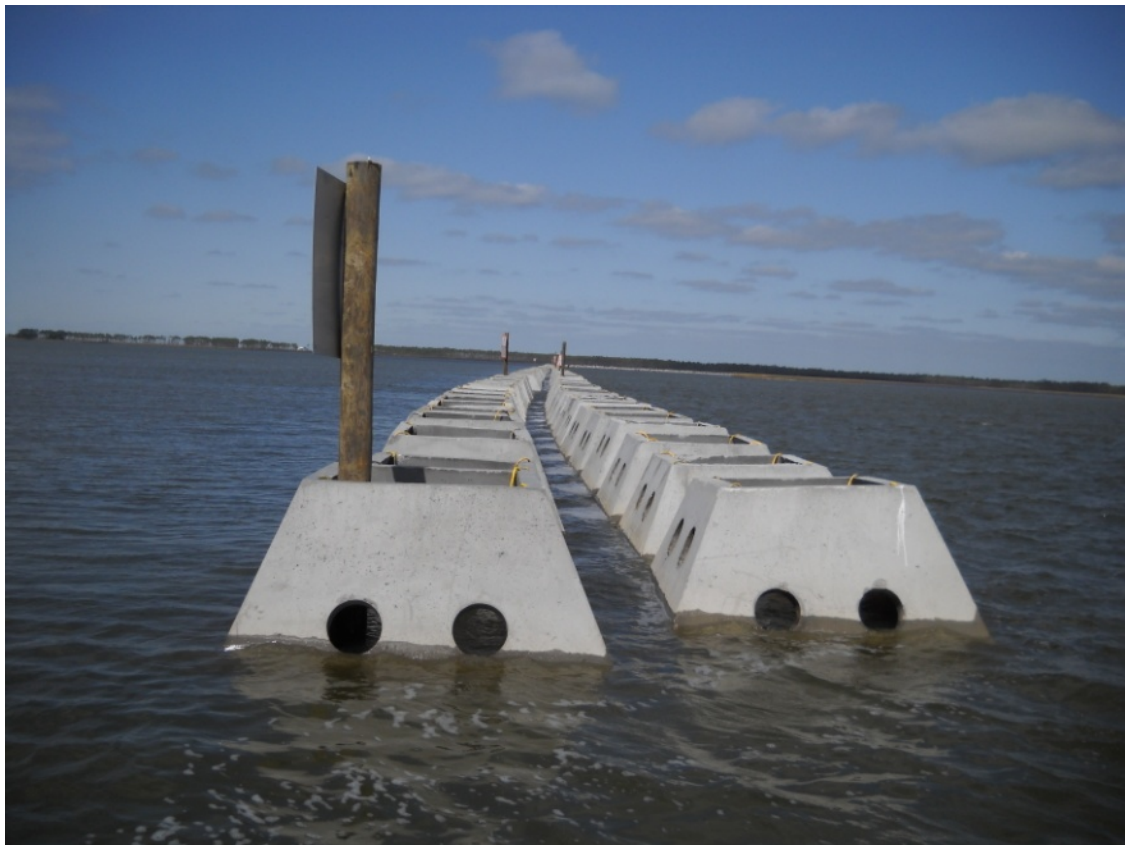
Figure 10. Water-level photograph of the Little Bay Project breakwater during construction before sediment pumping and vegetation planting. This photograph shows the end of one of the 61-m long breakwater sections taken from in one of the 12-m long gaps in the breakwater.
