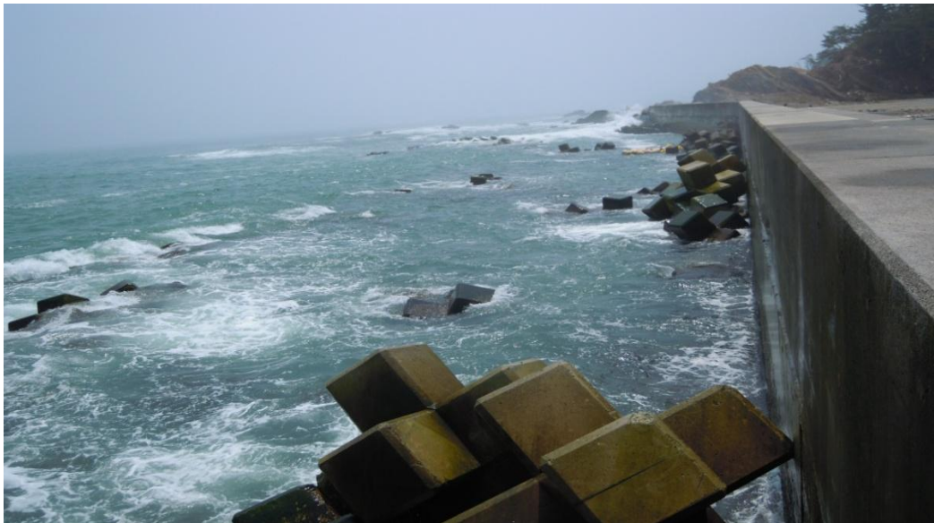
Figure 2. Failed X-Block Armour Units at Hikado Port
