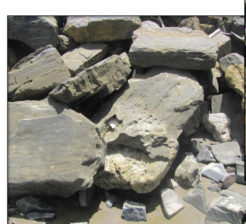
Weathering of the local "Blue" Limestone used to construct the revetment
