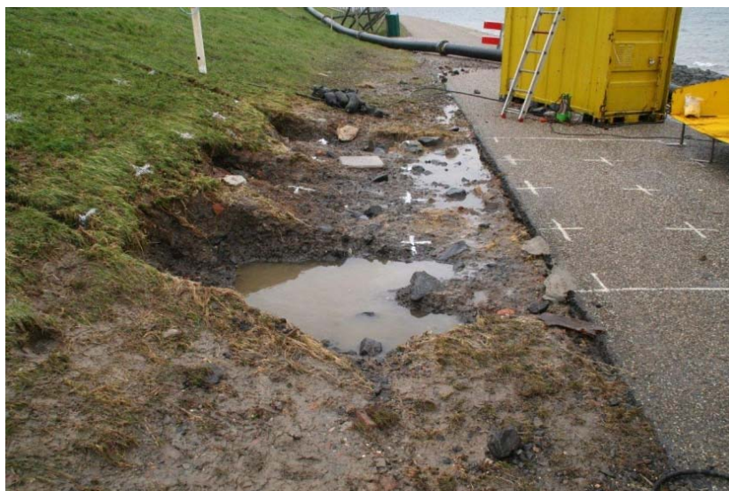
Figure 13. Final damage after the pilot run-up test.
