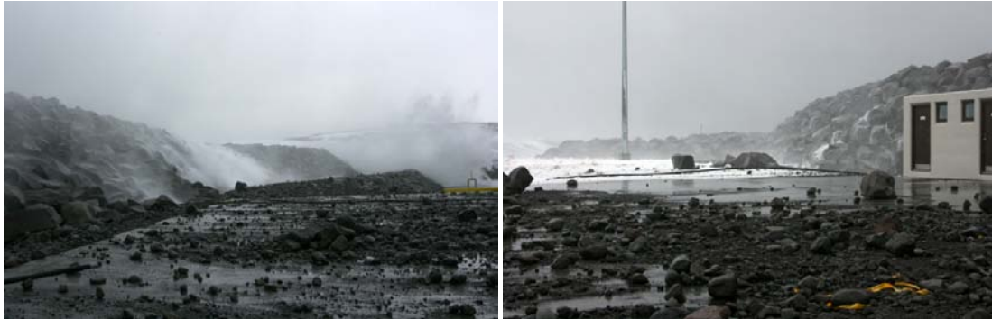
Figure 16. Husavik berm breakwater at the end of the 25 October 2008 storm. Gravel and small rock from unpaved area behind the crest washed upon the quay area.
