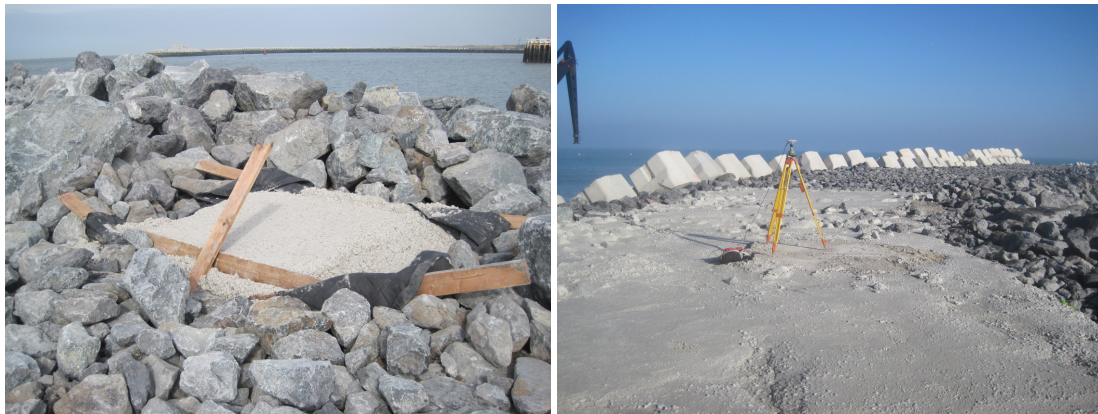
Figure 18. Pictures of settlement block poured in the breakwater (left) and set up of a total station to measure settlements (right).
