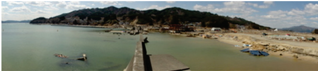
Photograph 6. Broken seawall facing to Funakoshi Bay at South of Funakoshi Area. The height of the seawall was 7.4m above mean sea level.
