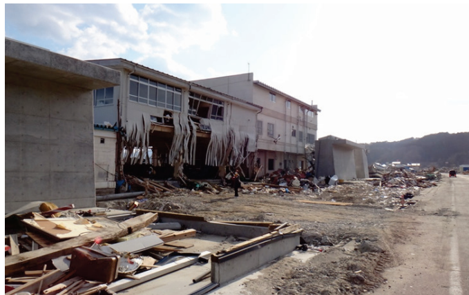
Photograph 3. Gap between new seawall segments at Osawa Fishery Port of Yamada Town. The tsunami flowed into the residential Osawa Area through the buildings of Osawa Fishery Port.
