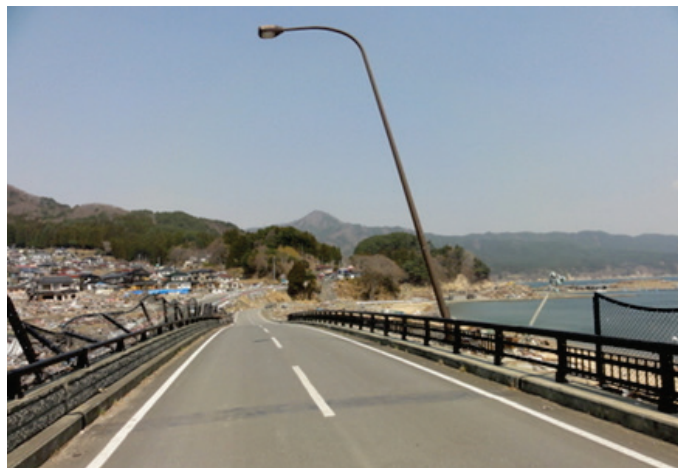
Photograph 9. At the top of the overpass, the lighting post and parapets were bent landwards, which is attributed to dominant inflow during the runup phase.
