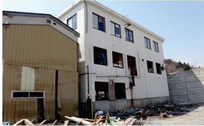
Photograph 5. An inundated building just outside the new seawall of Yamada Fishery Port of Yamada Town. A clear mudline watermark, slightly above the top of the second-floor window frames, indicated a tsunami height of 8.7m, more than 2m higher than the seawall.
