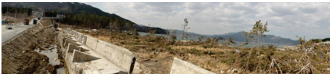
Photograph 7. Coastline facing to Yamada Bay at North of Funakoshi Area. The seawall and trees collapsed in northern direction (right in the photograph) indicating a northward directed main tsunami force.
