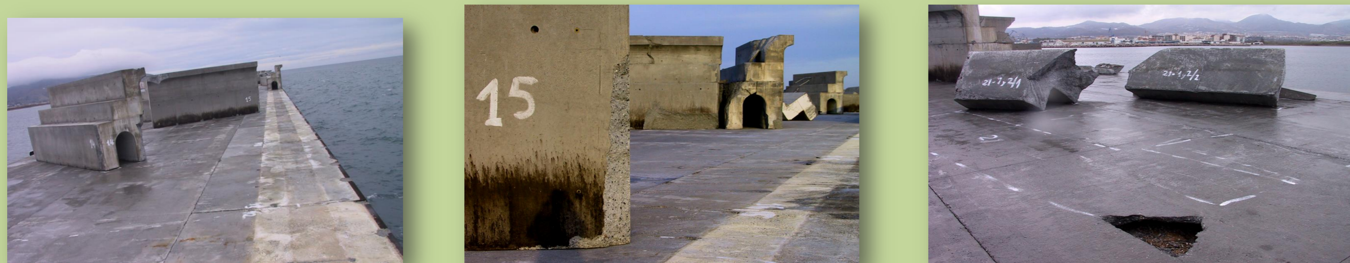
Figure 1: Damage generated in the vertical breakwater during the storm event in Motril
