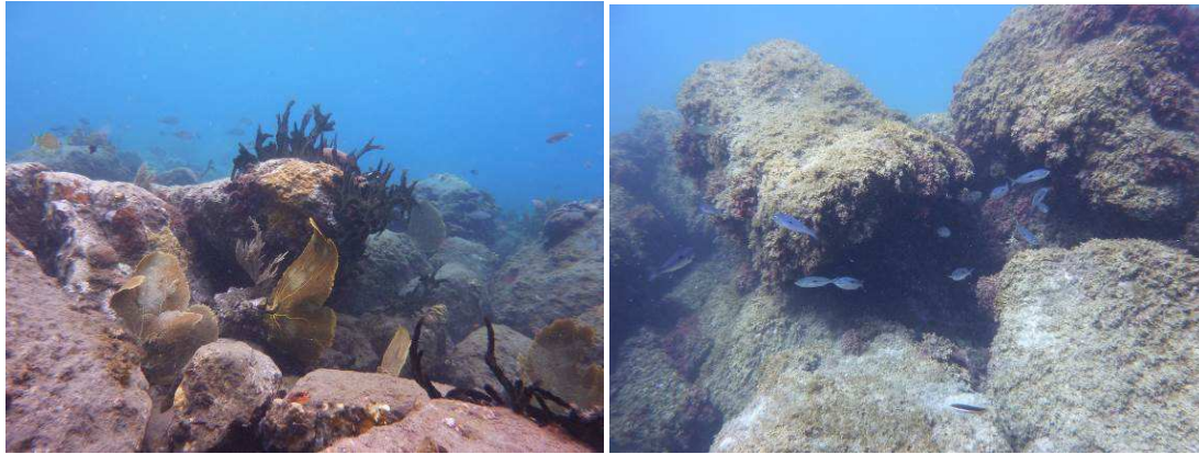
Figure 15. Toe reinforcement in Case Pilote (Martinique) (left) and toe berm reinforcement rocks in Pointe Rouge covered of algae (south of France)(right).
