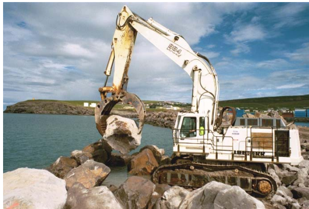
Figure 4. A 110 tonne excavator working on a level of Class IV rock of 1 to 4 t rock, placing Class I of 16-30 t at the head of the Husavik berm breakwater, Iceland.
