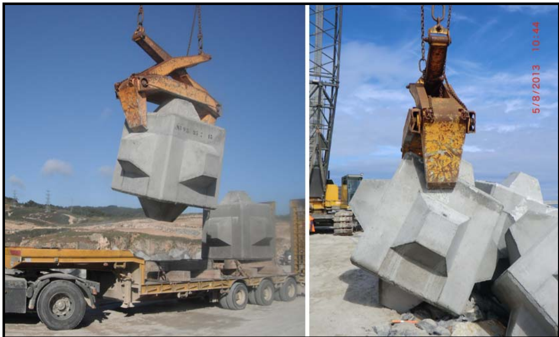
Figure 9. Single pressure clamps handling and placing Cubipod units on the armor slope.
