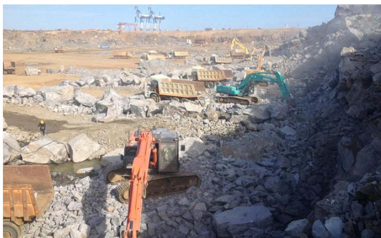
Figure 9. Extraction of the slightly weathered rock in the harbour basin area down to a final level of -17 m.
