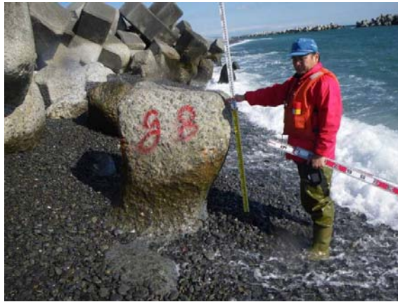
Figure 5. Erosion of concrete blocks settled on Suruga coast.
