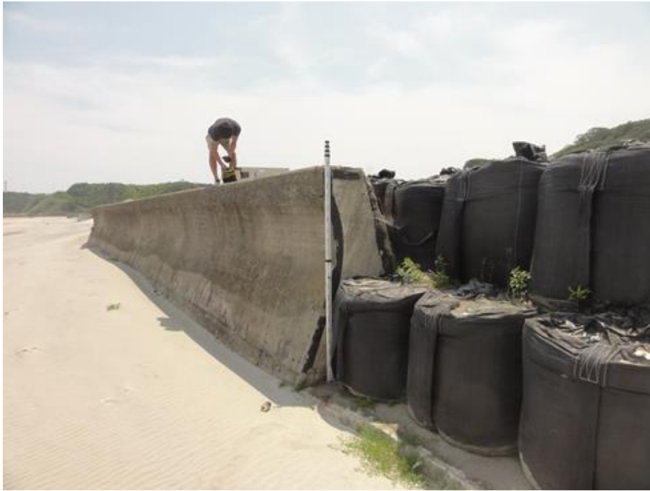
Figure 10. Damage of seawall parapet in Usuiso. The height of the parapet is about 2 m. The seawall was broken at the joint between the parapet and the basement. Black sand bags were placed as temporal recovery.
