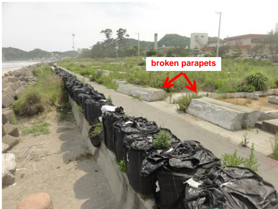
Figure 11. Damage of seawall parapet in Toyoma. The seawall was broken in the middle of the parapet. Broken parapets were transported inland. Black sand bags were placed for temporal recovery.
