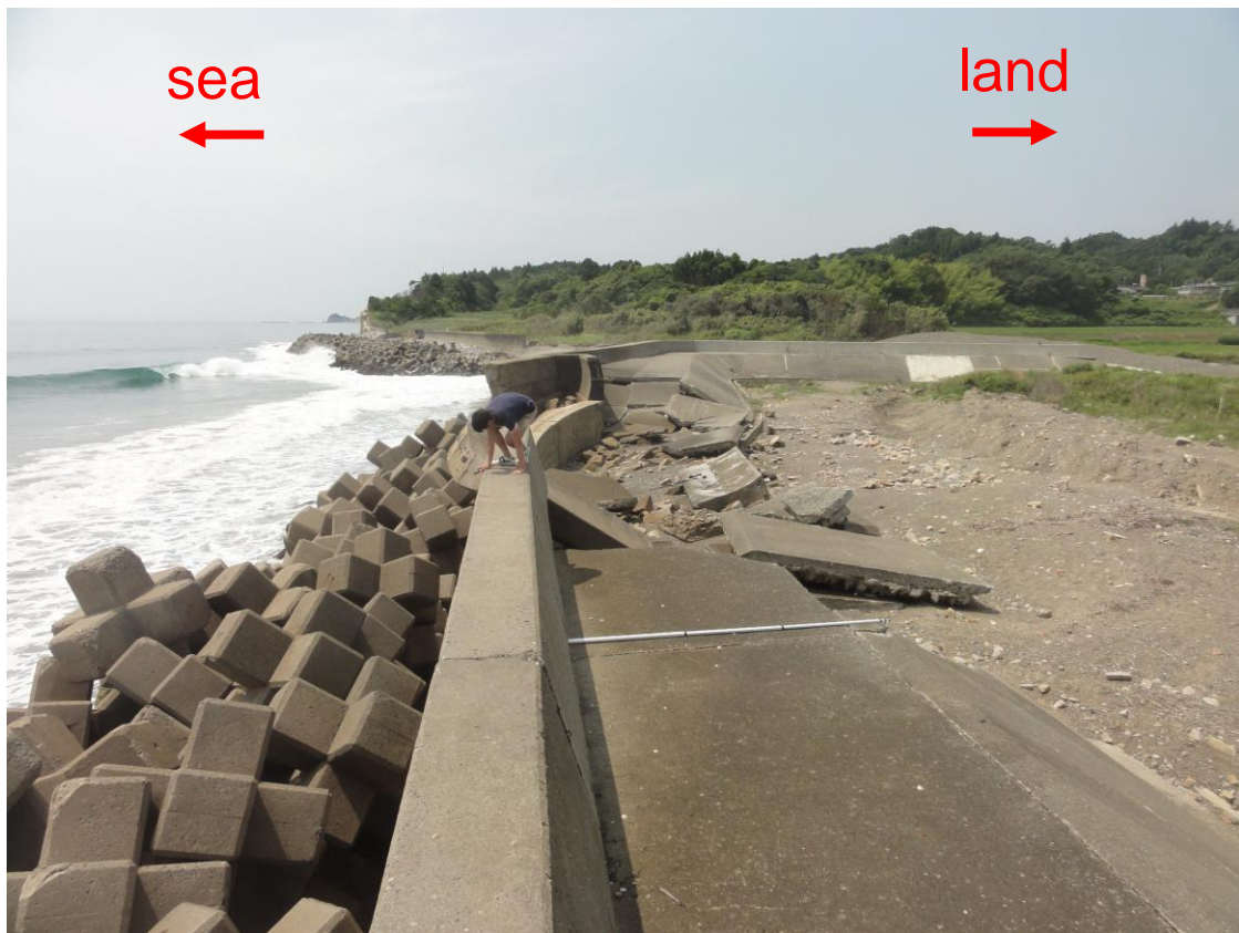
Figure 8. Damage of seawall in Oriki. The parapets with 1.5 m height were broken and transported about 50 m inland. A large scour hole is observed behind the seawall.
