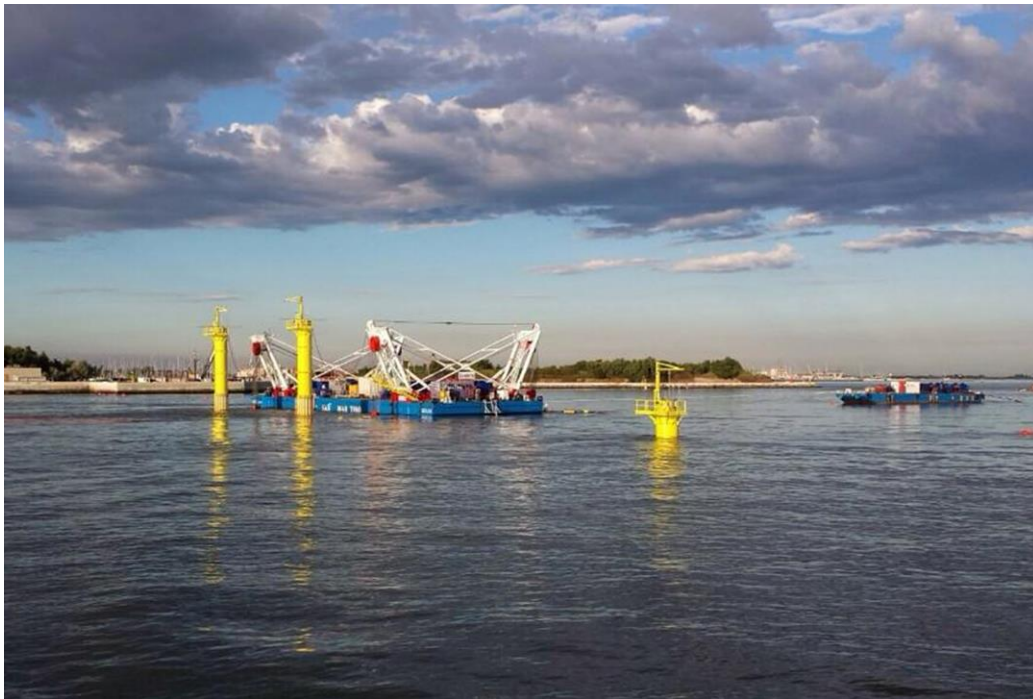
Figure 1. Golia pontoon placing a gate caisson for the Venice flood barrier at the Chioggia inlet.
