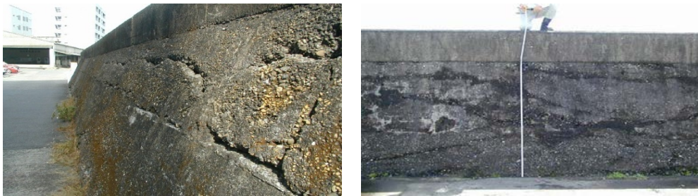
Photo 2. A concrete of the seawall becomes aging (Originally constructed around 100 years ago)
