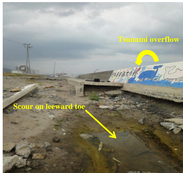
Figure 2. Damaged seawall at Ishinomaki port.
