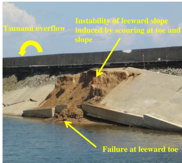
Figure 5. Damaged structure at Soma city.
