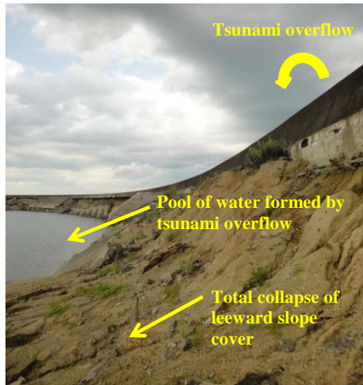
Figure 4. Damaged structure at Watari town.
