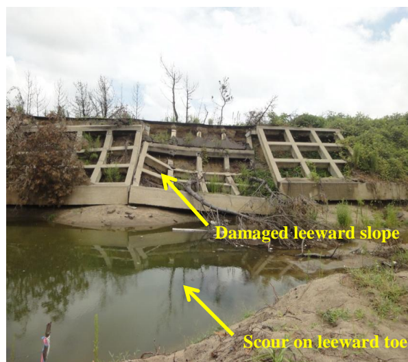
Figure 3. Damaged structure at Iwanuma city.
