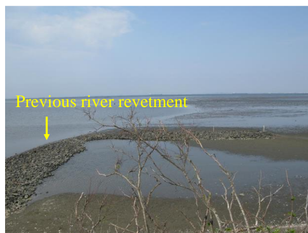
Figure 5. Photograph of L-shaped revetment, taken from the top of the mound immediately north of Obitsu River mouth.
