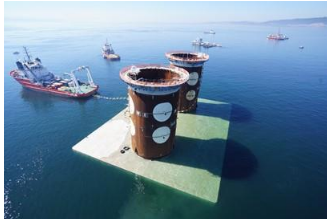
Figure 1. Floating of a caisson for submerged foundation of Korfez Suspended Bridge in Turkey.
