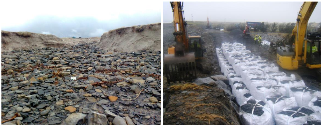
Figure 1. Breach in dunes system in the north (left) and emergency repair work being undertaken on the coastal embankment in the south (right) .Photographs provided by Clare County Council.
