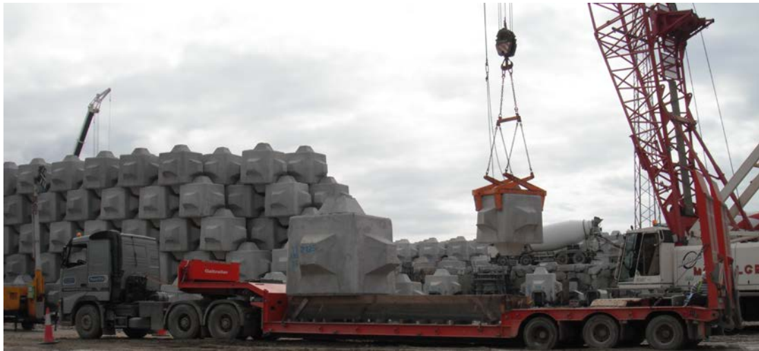
Figure 8. Loading Cubipods onto flat bed platform truck to be transported to the placement site.
