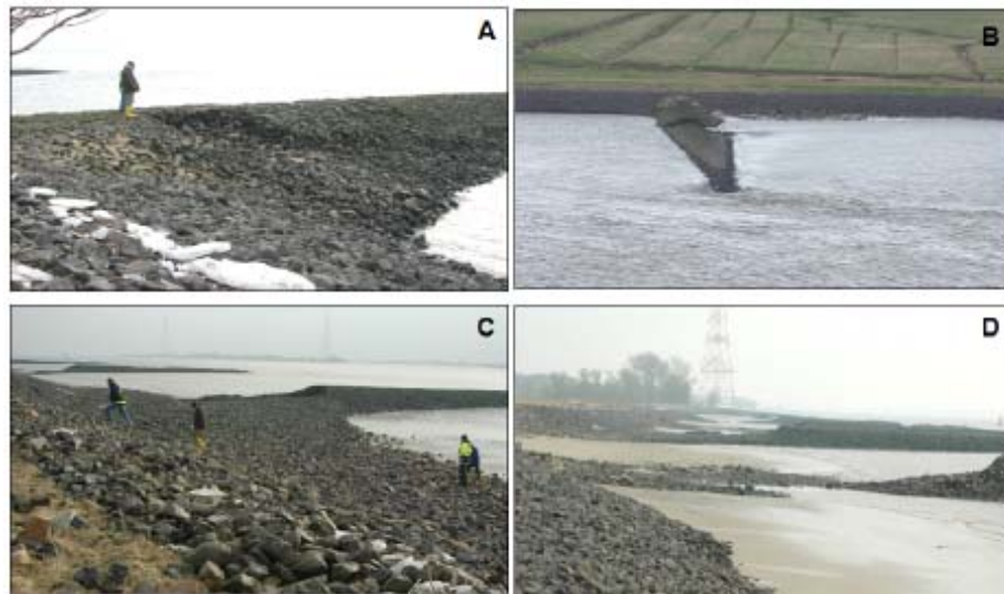
Figure 1. Damage development on groins at Juelssand, Unterelbe (BAW 2012)
