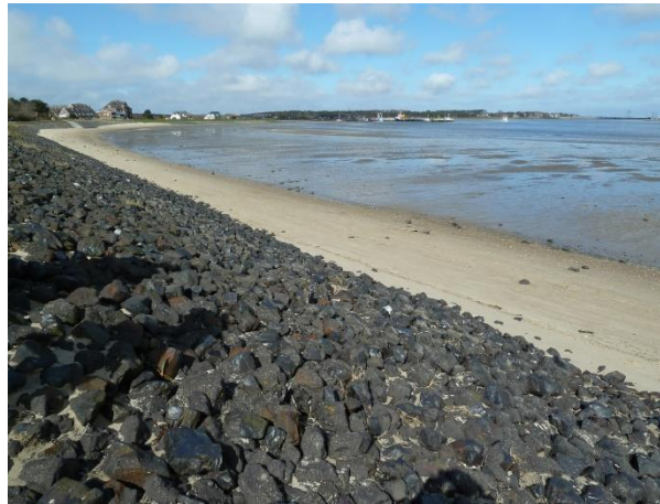
Figure 6. Coastal protection slope using Elastocoast technology on Amrum inland in the North Sea
