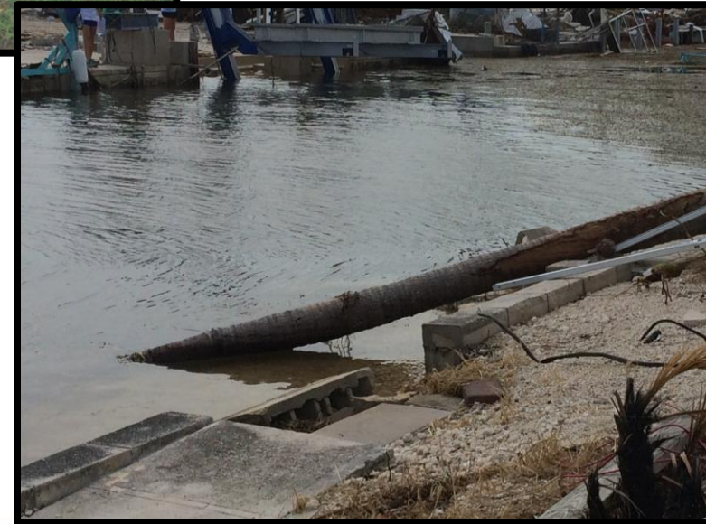
Bulkhead: cracks, undercutting, collapse
