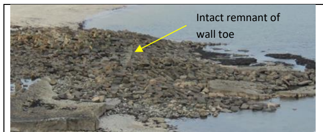
Figure 4 Collapsed breakwater, Skateraw, East Lothian, Scotland
