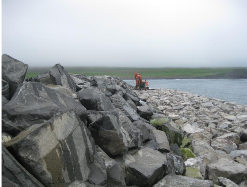
Figure 7. Ground level photograph of completed Phase 2 repairs (Photo courtesy of Brice Construction).
