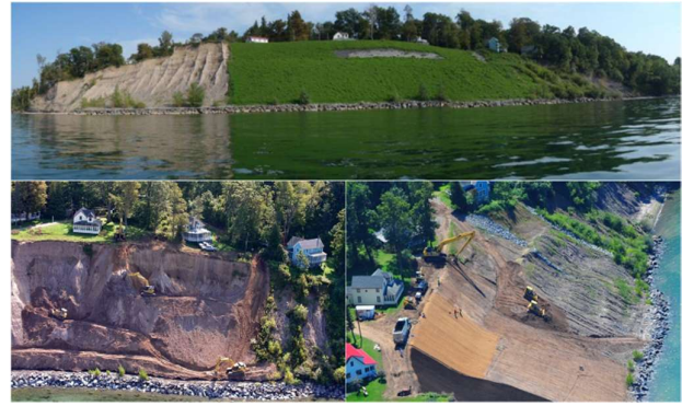
Figure 6 - (Counterclockwise from bottom left), Initial excavation, Coir mat installation, Final stabilized shoreline, Lake Ontario, New York
