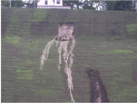
Figure 4 - Localized sluffing caused by Perched Groundwater
