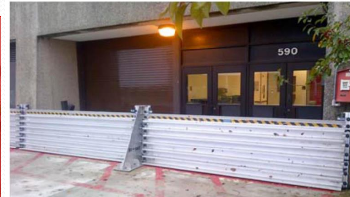
Figure 6: Temporary flood protection stoplogs installed at the U.S. Naval Academy (Source: U.S. Navy)
