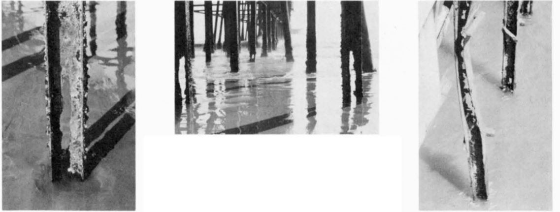
Fig. 1. ABRASION IN BREAKER LINE
