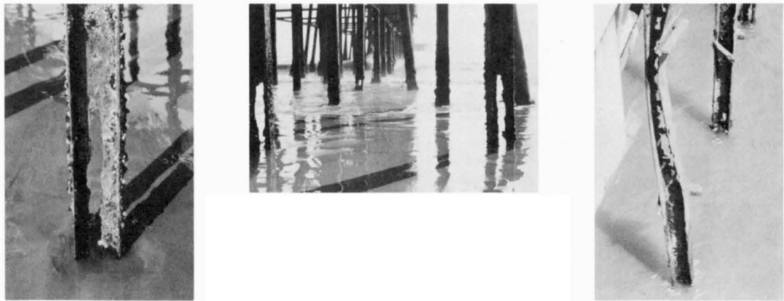
Fig. 1. ABRASION IN BREAKER LINE
