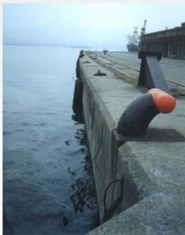
Damage on quay wall in Derince Port after Kocaeli Earthquake (1999), in Turkey
