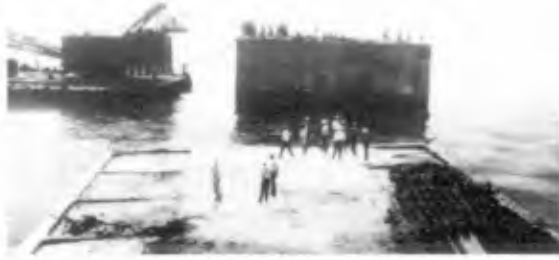
Figure 8. Installation of an "Island" caisson, which is aided by a pre-anchored 80 MT pontoon
