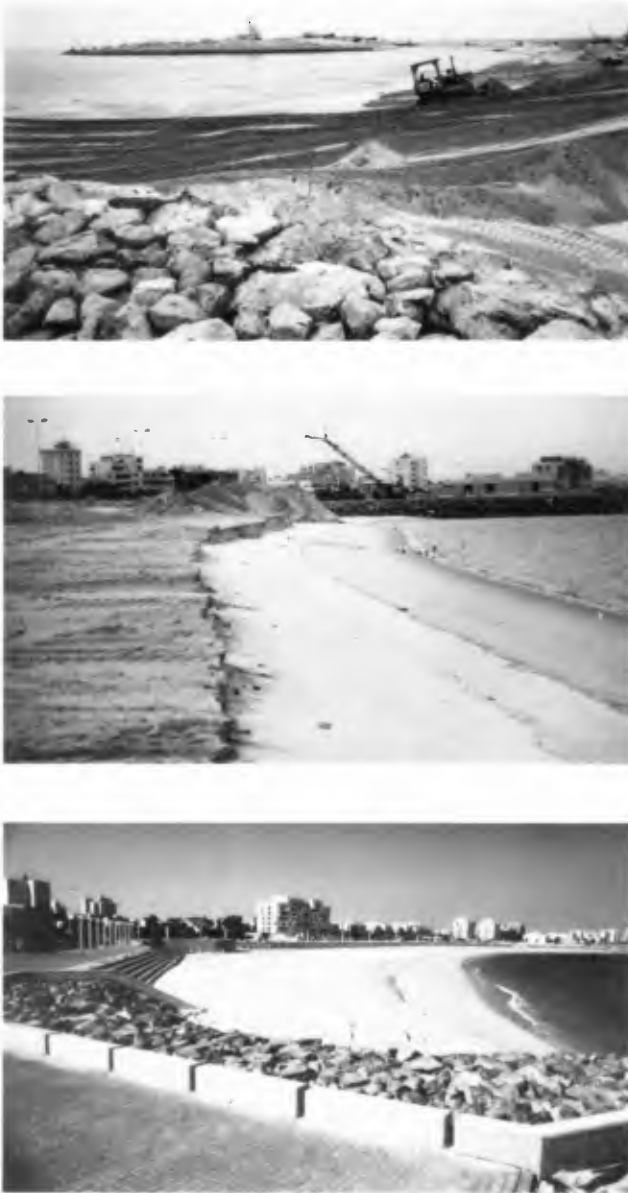
FIGURE 5. Stages of beach construction by land-based equipment beginning with spreading along the profile (top), natural adjustment of the beach face (middle), and final completion in an equilibrium planform (bottom). Photos taken at low tide in March 1985 by T.W. Kana.
