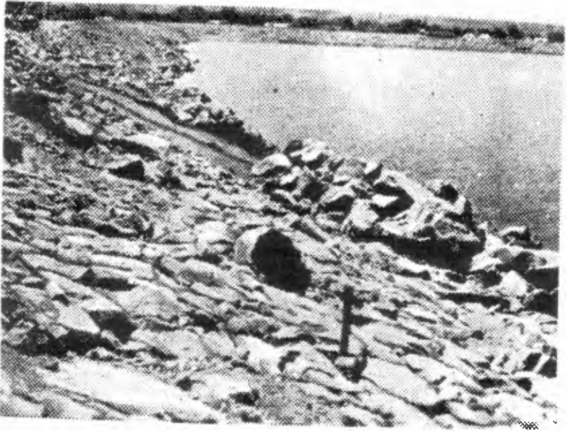
Fig.3a) Upstream slope of the Kamensk dike during the rock toe repair
