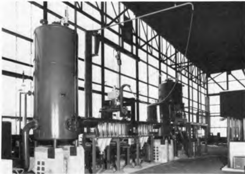
The DHL wave tunnel
