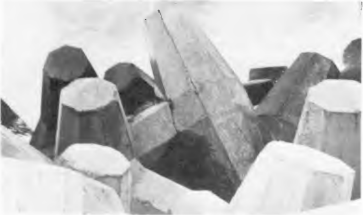
b. Broken reinforced dolos
