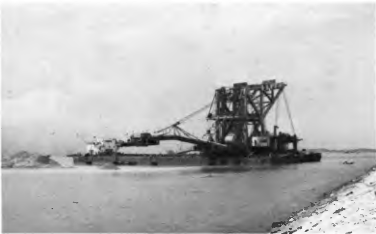
Plate 6. Reclaimer unloading fill material from barge into the sea to form reclaimed land.
