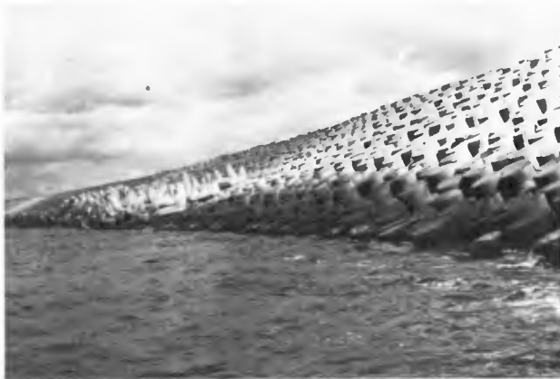
Tribar and DoLos revetment, Port Botany, New South Wales
