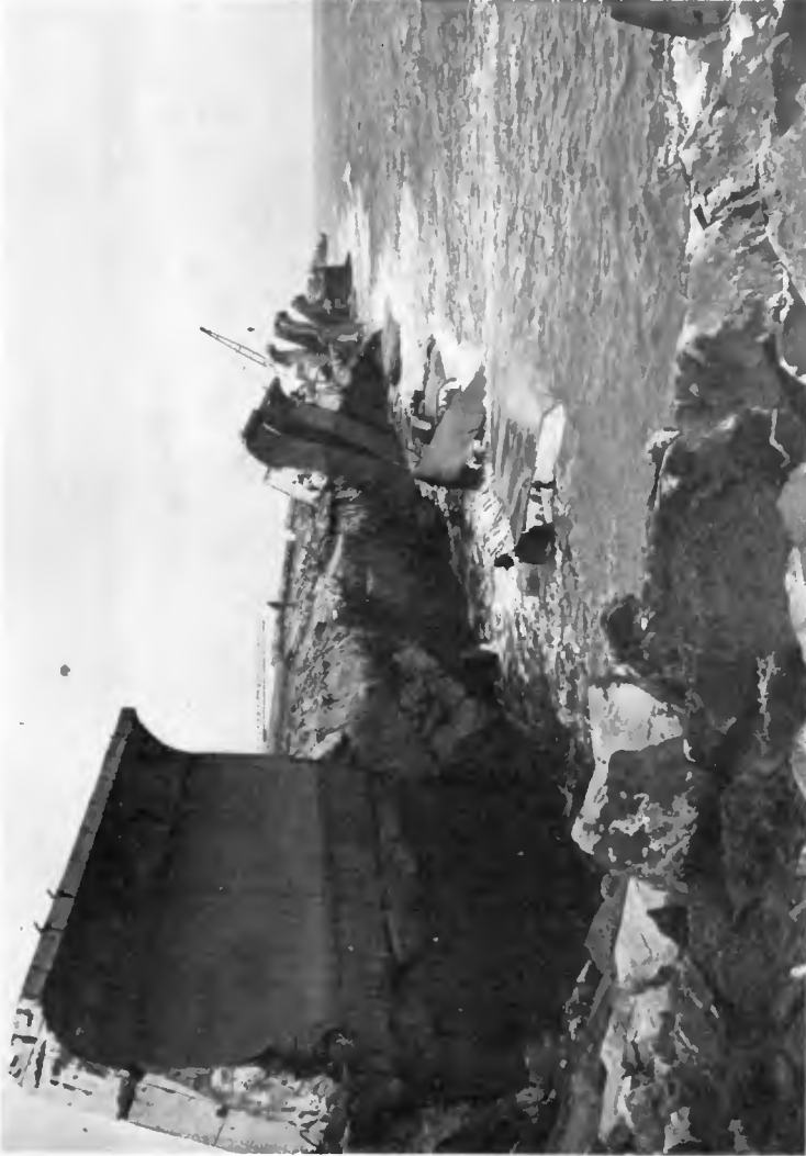
Figure 1 Damage to the seawall and dolos, taken immediately after the February 1978 storm (photo from GAS)
