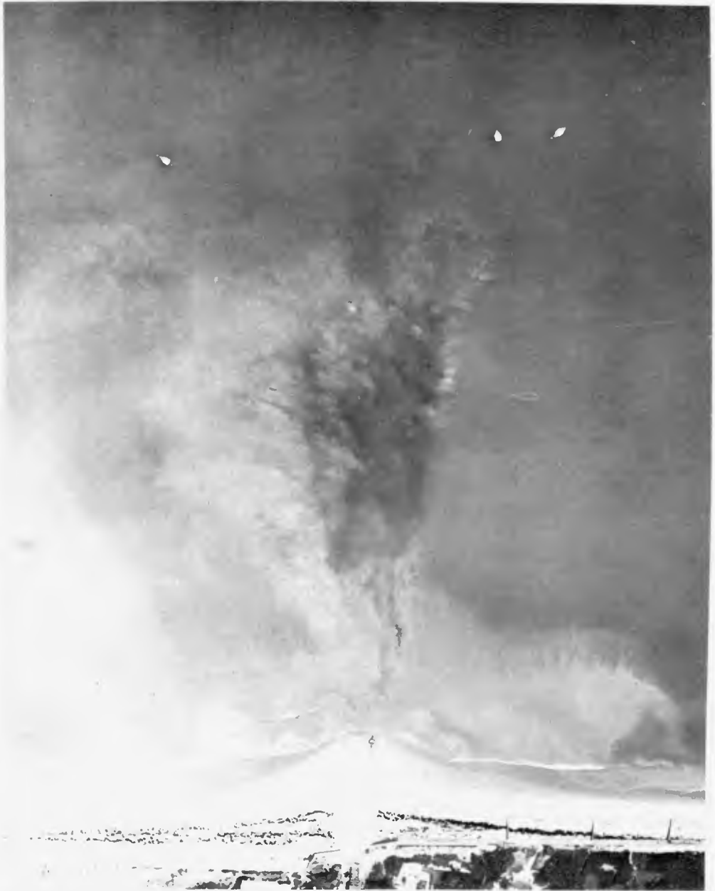
Photograph 3. Drag Scraper in Action. Note the large amount of suspended sand in borrow area.
