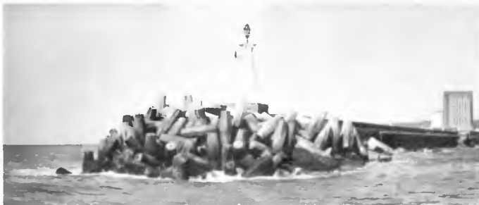
Fig. 3. Breakwater head protected with 19-3/4-ton Dolosse.
