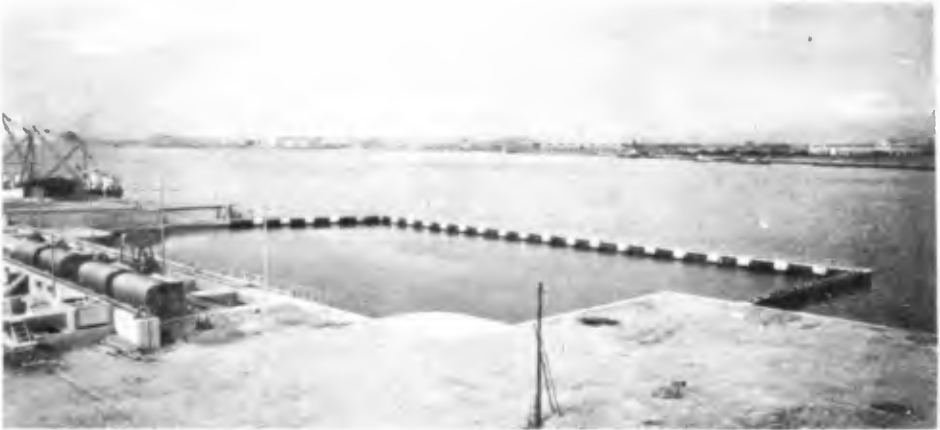
Fig. 11. A view of curtain-wall type bottom-water intake for Sakai-Port Thermal Power Station (Kansai Electric Power Company).
