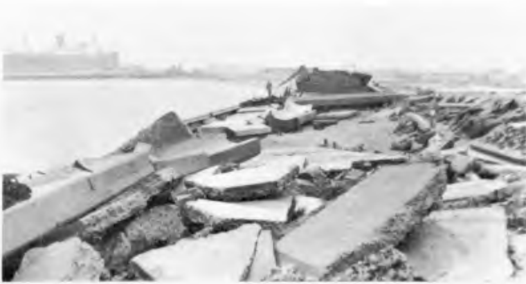
Photo.4.3 The damage of Isozu coastal dike.
