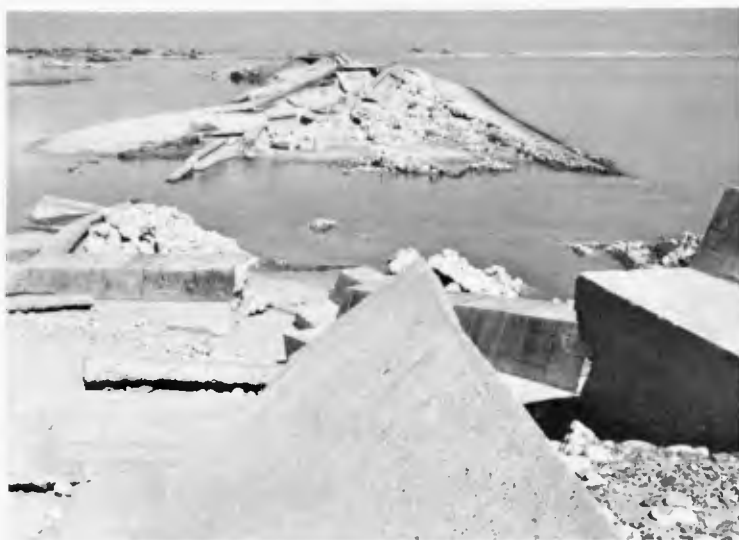
Fig. 1-2 Disrupted embankment near Kuwana City
