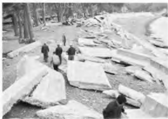
Fig. 2-7 Completely covered structure collapsed from settling of sand filling for a length of over 100m as partition wall was lacking. (Port of Nagashima)
