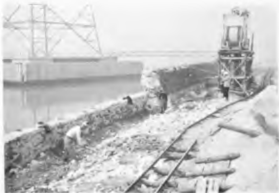
Fig. 2-5 Wall behind power transmitting tower remained in a little damage. (Port of Nagoya)
