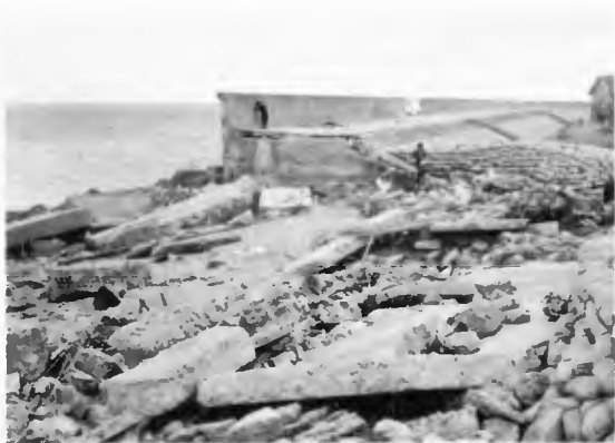
Fig. 2-8 Right side of the wall was saved by partition wall. (Yokkaichi City)
