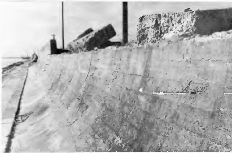
Photo.4.5 The overturning of parapet in the coastal dike at the left side of Nikko River.
