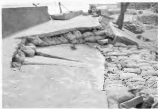
Fig. 2-6 Wall smashed by waves as interior was in a hollow state from settling of sand filling. (Yokkaichi City)
