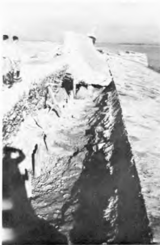
Photo.4.4 The damage of Koeishinden coastal dike at Handa.
