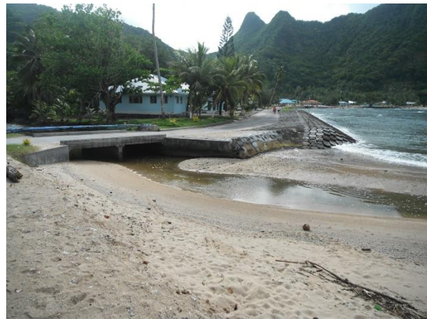
Figure 1 - Stream outfall and low-lying coastal highway in American Samoa
