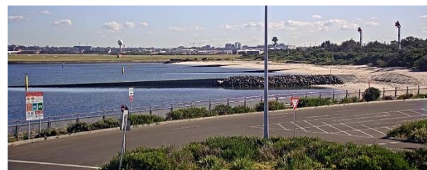
Figure 5 - Rock work encapsulating storm water drains (nearest and farthest groynes). Yellow marker piles denote the midpoints of the submerged fibre-reinforced plastic sheet piling groynes
