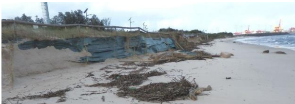
Figure 1 - Foreshore Road Beach erosion 5 June 2012
