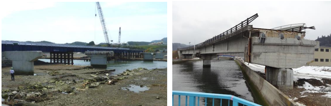
Figure 1. Damaged bridges after the 2011 tsunami in Japan: (a) Koizumi bridge on the left (from EERI Report 2011) and (b) Utatsu bridge on the right (from M. Yashinski)
